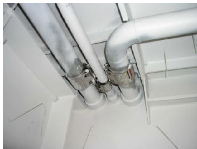
Space saving pipe lay out
